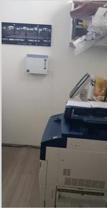
iTherapy 1 installed near the printing press
